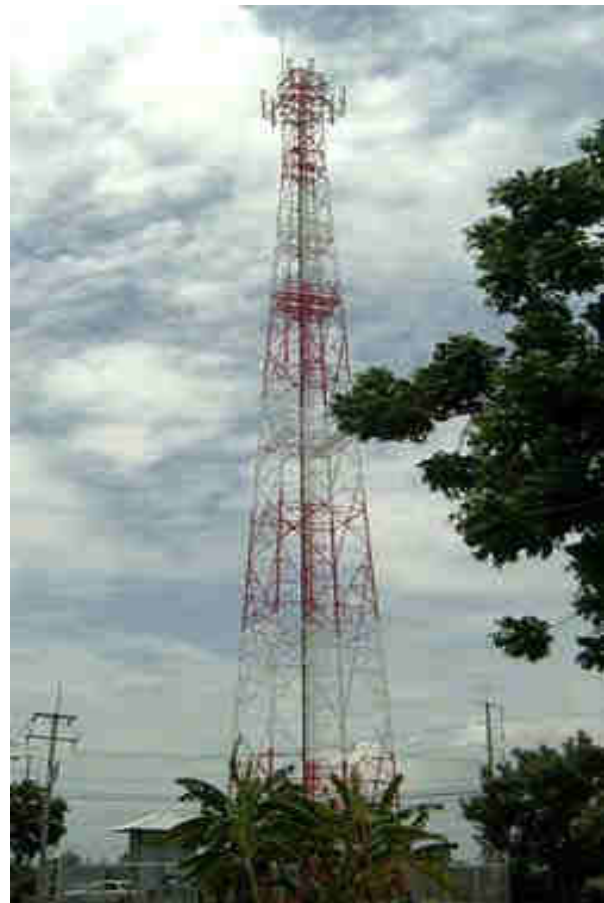
Fig. 1.1: Wattana Transmission Tower
